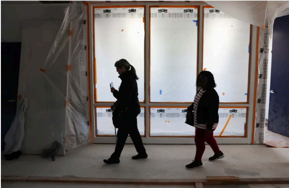
Asian American Pacific Islander Coalition of North Bay vice president Grace Cheung-Schulman, left, and CEO of North Bay Black Chamber of Commerce Nancy Rogers tour the second floor of offices under construction at BOSS in Santa Rosa on Wednesday, January 14, 2026. (Christopher Chung/The Press Democrat)
